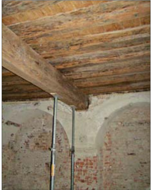
17. Gotycki strop z XVII-wiecznym podciągim w sali na parterze ratusza. 17. Gothic ceiling with a seventeenth-century binder in a chamber on the ground floor of the town hall.
