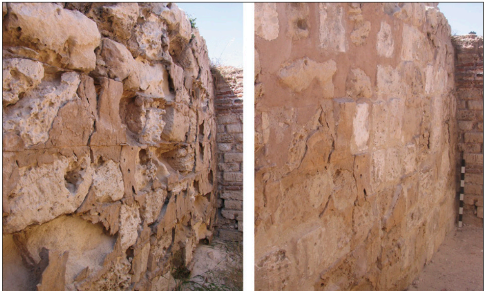
Fig. 22. North wall of the cistern: left, before, and right, after conservation (Photos G. Majcherek)
