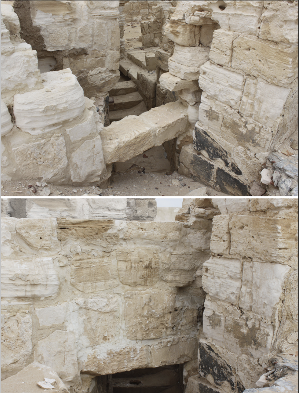
Fig. 11. Southern Bath. Wall above the passage to the underground corridor (between rooms 18 and 8a), before and after continued restoration in 2014 (Photos R. Czerner)
