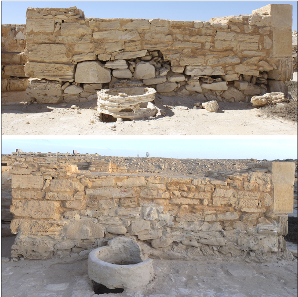
Fig. 14. Courtyard wall in house H9 before and after conservation, exemplifying the scope of maintenance repairs (Photos R. Czerner, W. Grzegorek)
