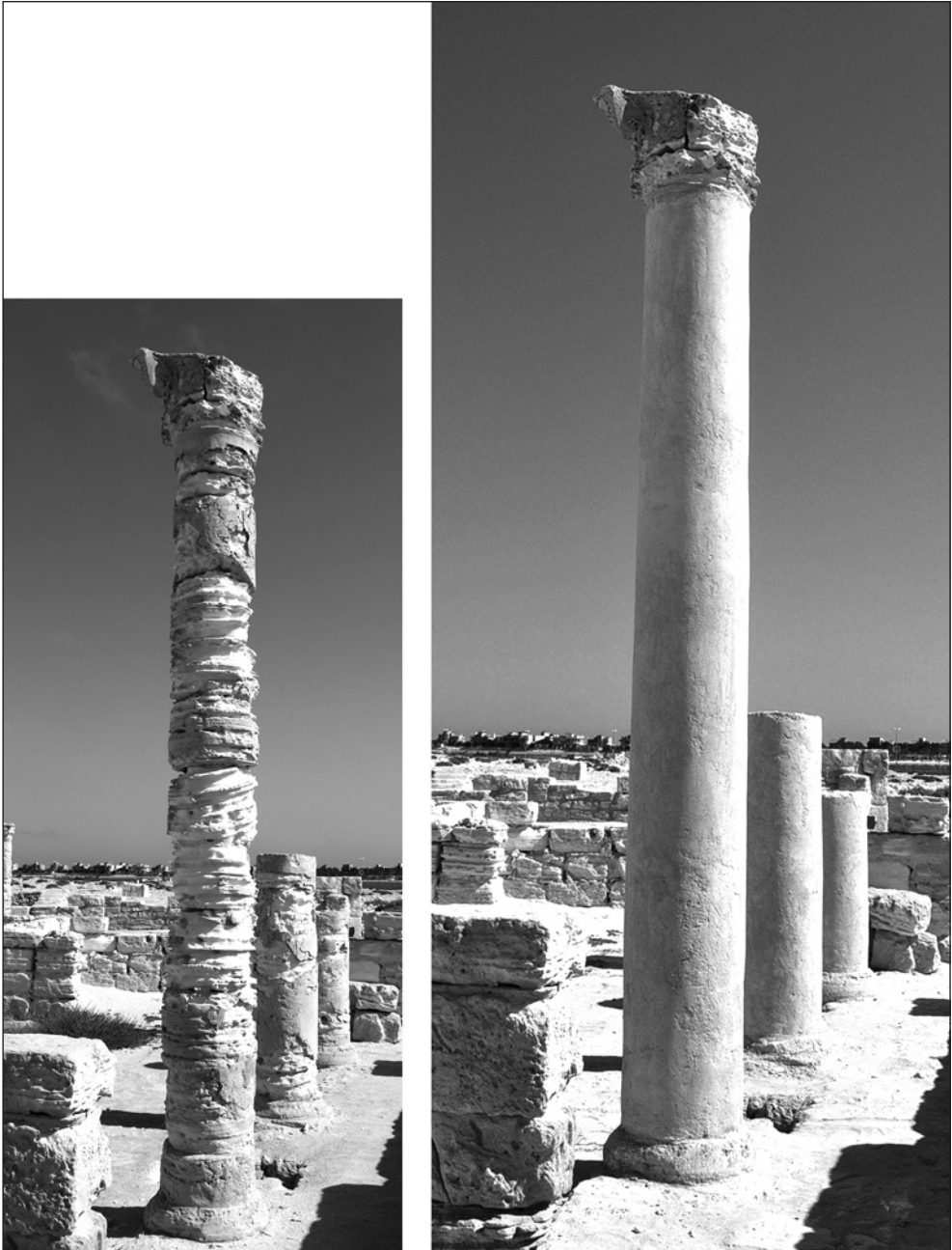
Fig. 5. House H10a. Damaged columns before conservation in 2012 (left) and after (Photos R. Czerner)
