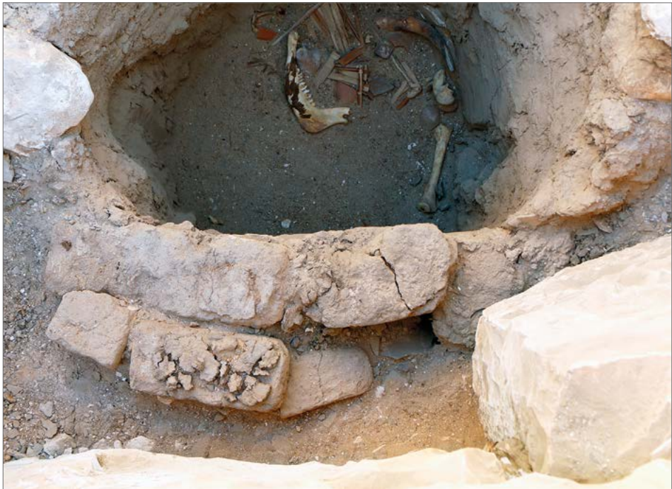
Fig. 7. Top of the east wall of the southeastern foundation pit, covered in its northeastern corner by part of a limestone foundation block (IFAO/PCMA UW/photo N. Beaux)
