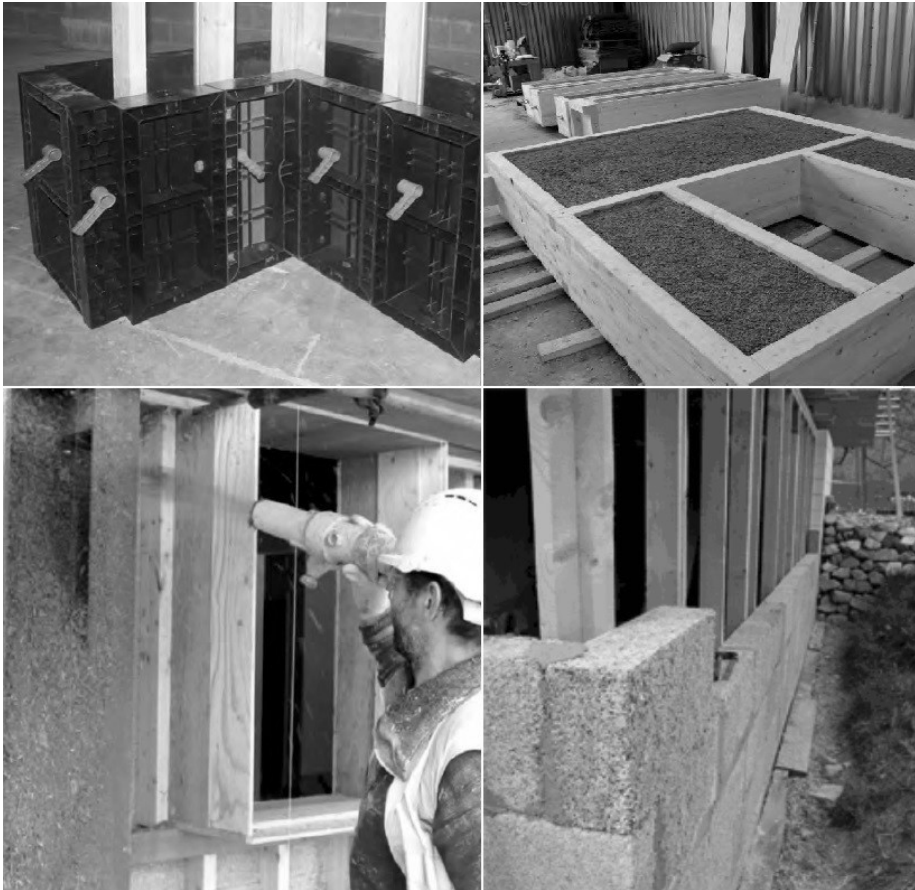
Photo 1. Hempcrete techniques: casting monolithic walls, prefabrication of the entire wall elements, spraying, bricklaying
