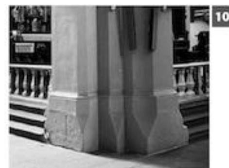
10. Kamieniec Ząbkowicki, the Cistercian church, the base of the pier in the eastern part.
