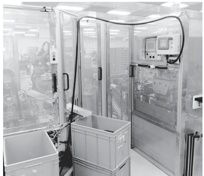
Photo 5. High frequency welder No. 2: a) before the shielding installation, b) after the shielding installation
