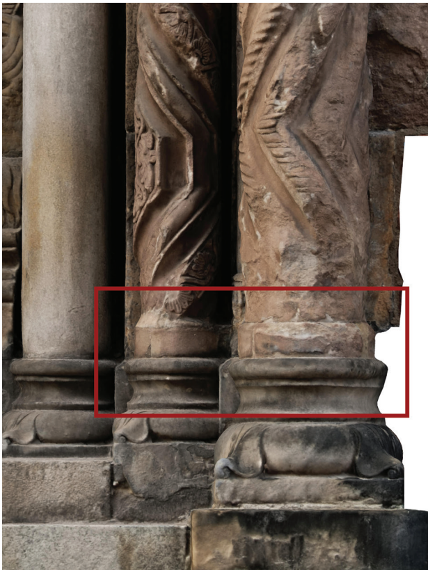
Fig. 7. The Olbin portal from the southern wall of St. Mary Magdalene Church in Wrocław. A fragment of photogrammetric inventory. Detail of the lower parts of the external columns of the eastern side. Cylindrical pads between the shafts and bases of the columns are visible (elaborated by F. Hackemer)
