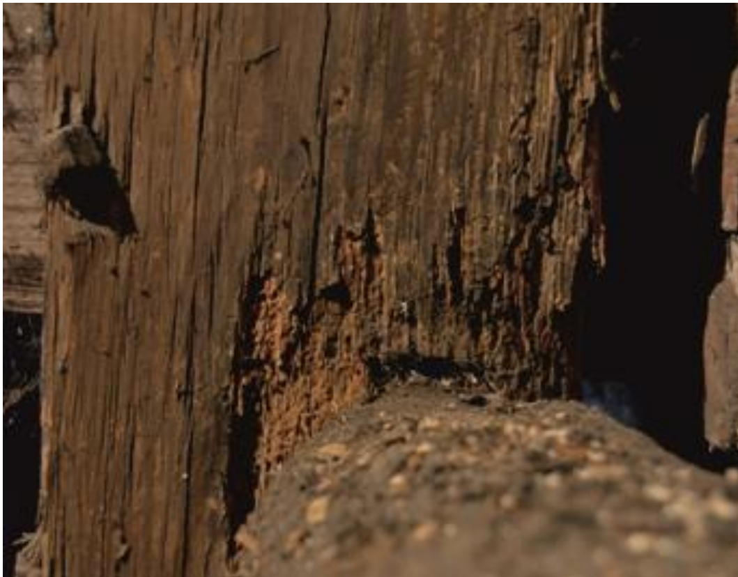
Fig. 9. Damage caused by insects Source: Own work.
