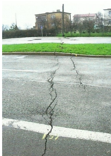
Fig. 6. View of damage to the road surface in the area of discontinuous linear terrain deformations Source: [10].
