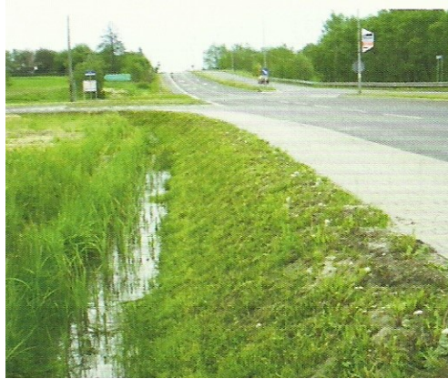
Fig. 3. Marginal reservoirs forming in roadside ditches in maximum land depression areas. The case where, after the formation of the depression basin, the culvert is not situated at the lowest point of the ditch bottom grade
