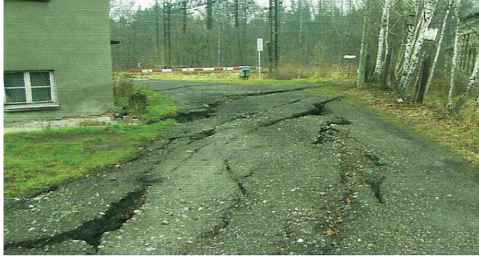
Fig. 22. Location of the PKP railway line no. 149 (CE-65) in relation to the range of discontinuous deformations Source: [10].
