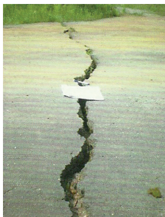
Fig. 21. Example of linear discontinuous road deformation of cement concrete pavement Source: [21].
