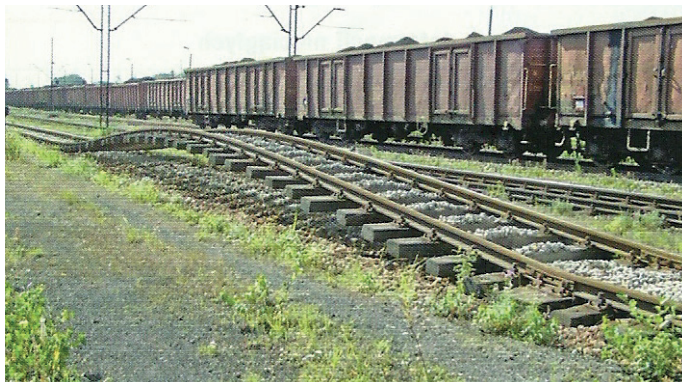
Fig. 24. Buckling of the track in the vertical plane as a result of superposition of horizontal deformations compacting the mining ground with thermal deformations of the track Source: [10].
