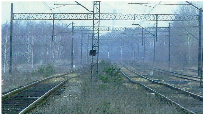
Fig. 23. Track discontinuous deformations as a local fault under the railway line PKP No. 149 (CE-65) Source: [10].
