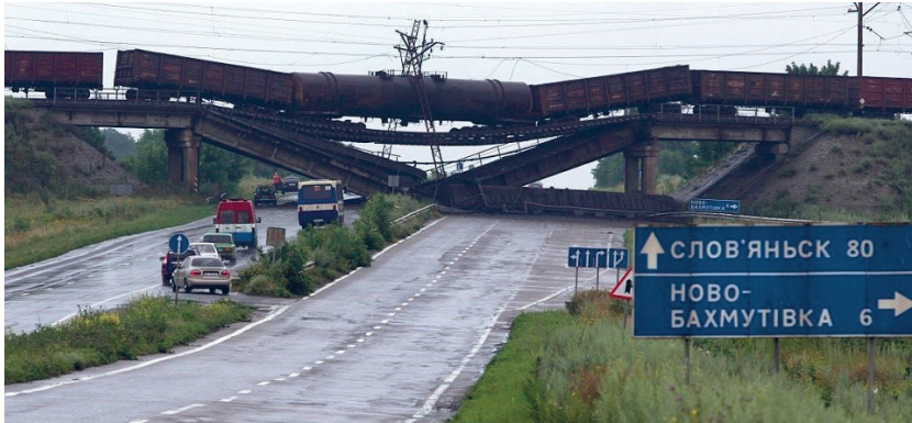
Fig. 1. Destroyed railway viaduct on the road near Novobakhmutivka (Ukrainian: Новобахмутівка) in the Donetsk region Source: [1].
