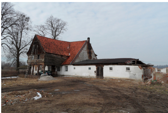
2. Kaniczki homestead (1757) before the translocation to the Olender Ethnographic Park in Wielka Nieszawka, state as in 2011
