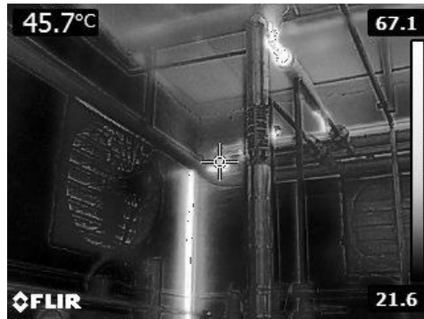
Figure 5. Thermographic picture of heat leaks in piping systems reaching 45.7 C°.
