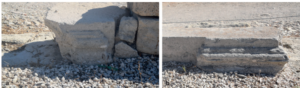
13. Counter-façade of the colonnaded hall: a. central entrance, pilaster on the south jamb; b. south entrance, pilaster on the north jamb (Phot. P. Pensabene).
